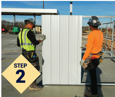
Attach the metal sidings onto the frame to provide a surface for the stone and brick.
